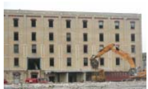
The symbolic building was reduced to a pile of rubble in just a few minutes (left). Fred Holdridge (bottom left) came all the way from German Village to see it. The big yellow building, however, remains while crews remove asbestos. Within the next few weeks, it, too, will be bashed, crushed, chopped, and scissored and be hauled away.
